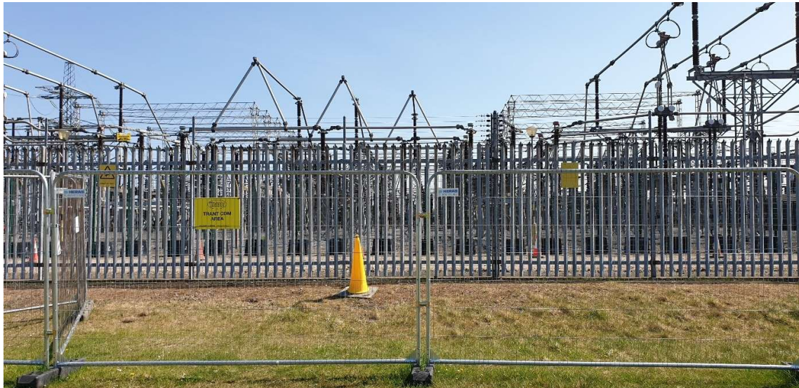
Photograph 4 – The existing 400kV National Grid Substation
