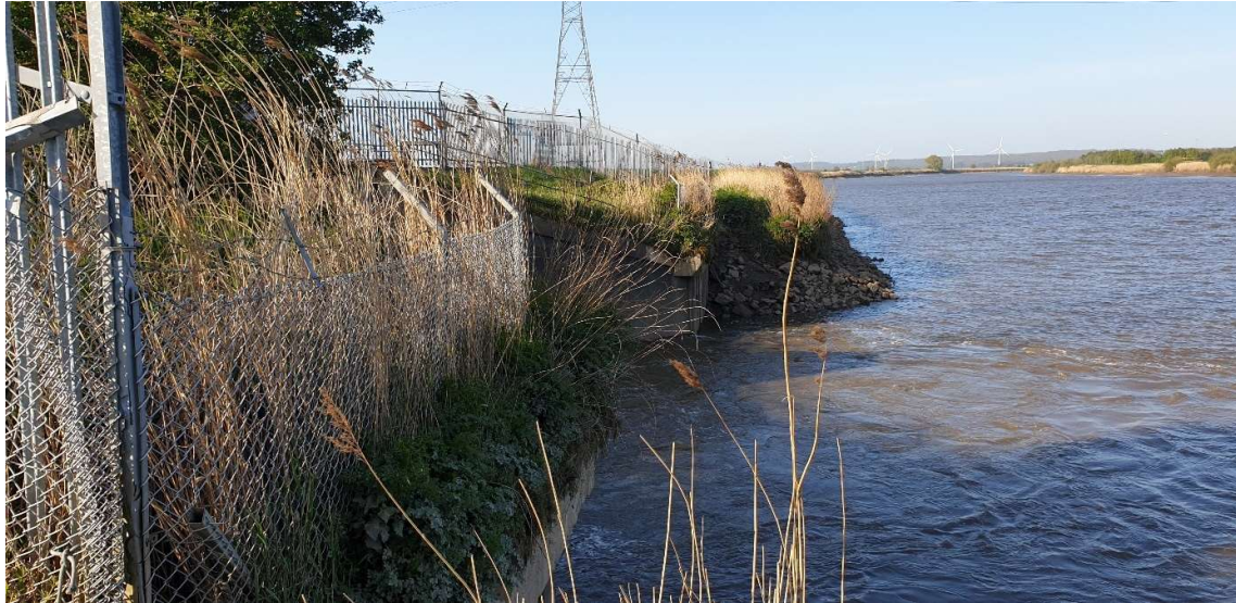
Photograph 7 – The existing Keadby 1 Power Station water outfall structure on the River Trent
