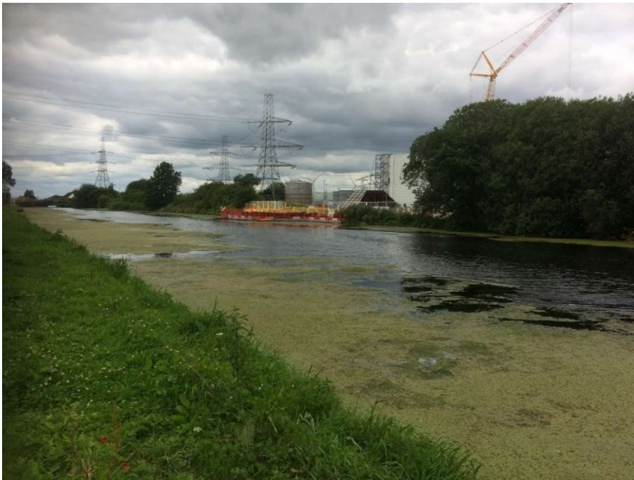
Photograph 22 – Stainforth and Keadby Canal looking towards the construction site for the Keadby 2 Power Station water intake
