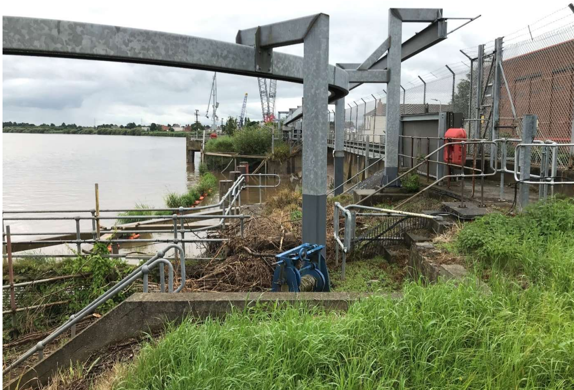
Photograph 6 – The existing Keadby 1 Power Station river water abstraction structure on the River Trent
