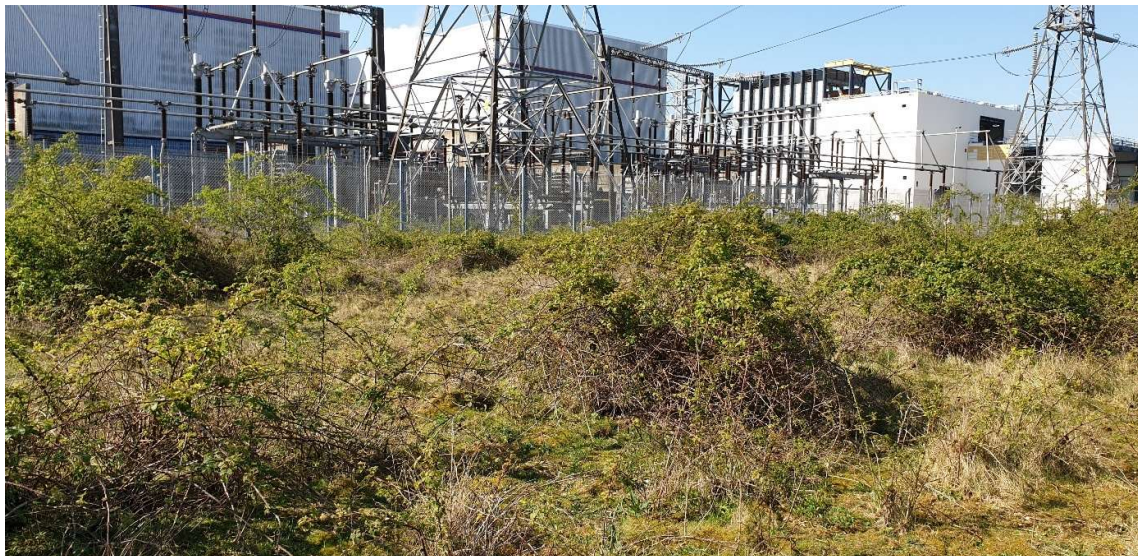
Photograph 18– Scattered bramble and rose scrub over rank semi-improved grassland, north of Keadby 1 Power Station
