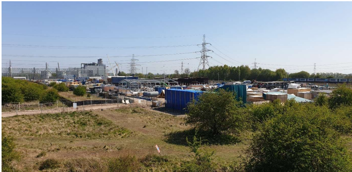
Photograph 3 - Keadby 2 Power Station Construction Laydown Area immediately east of the former Keadby Ash Tip
